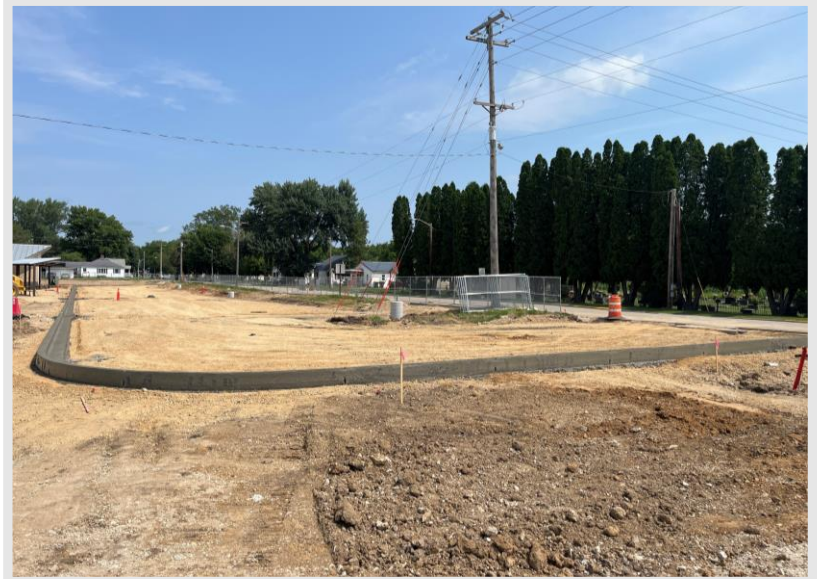
Curb and Gutter Poured in the East Parking Lot and Ready for Paving
