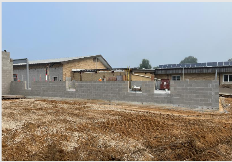
Area C Admin Offices Exterior Block Walls Placed and Waiting for Hydro Mobile to Finish Laying the Last Courses of Block
