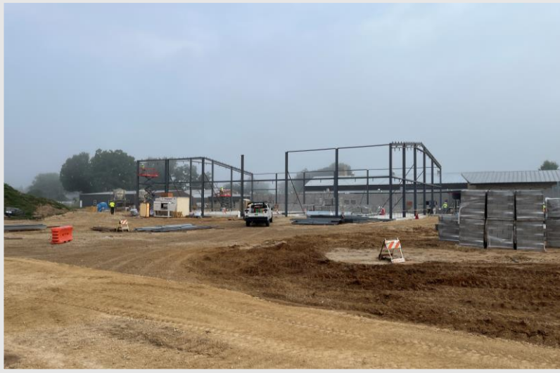
Exterior Sidewalls of the Pre-Engineered Metal Building in place awaiting the 105' Long Trusses
