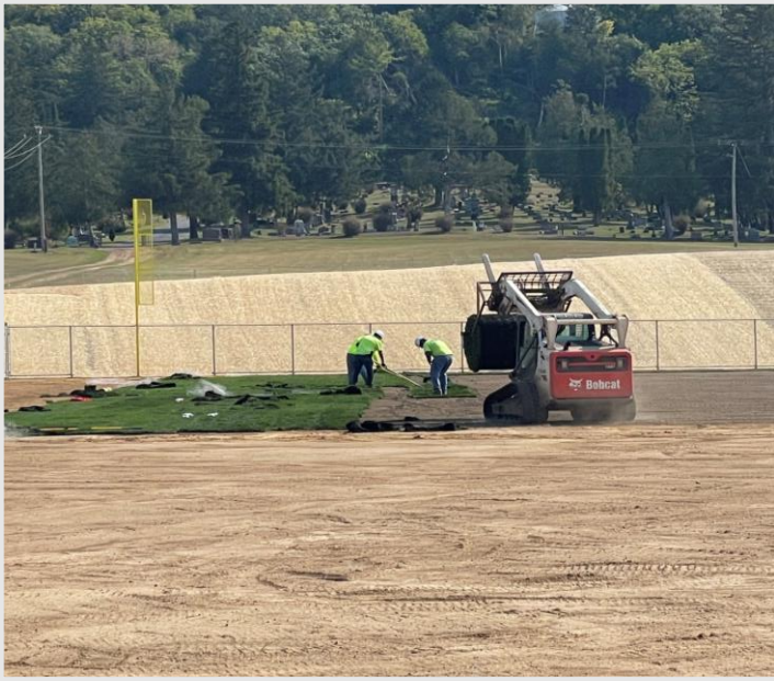
The new Ball Field has new Sod being laid in the Outfield.
