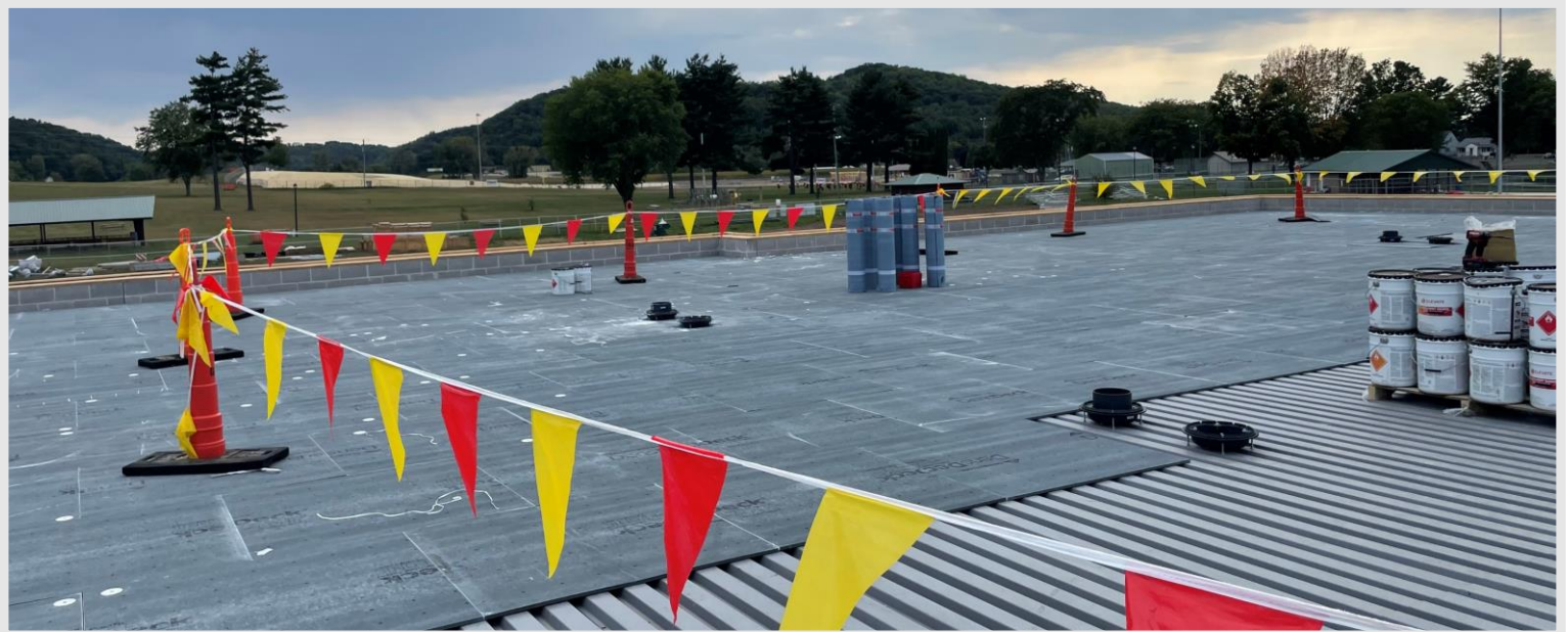
The Classroom addition is just getting its first layer of roofing material down before it add insulation and its EPDM Roofing membrane.
