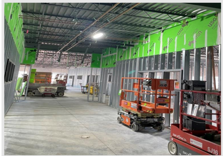
4 th and 5 th grade classrooms have been framed up in metal studs.
