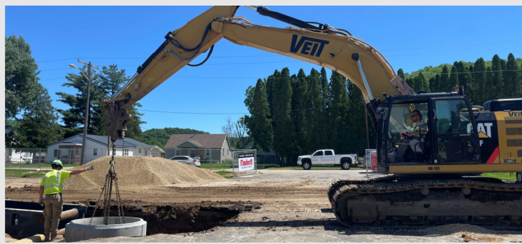
Veit's Site Utility Crew Installing a New Manhole in the East Parking Lot
